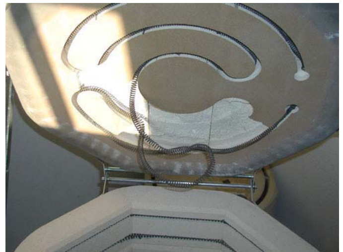
Collapsed kiln lid caused by thermal shock.
